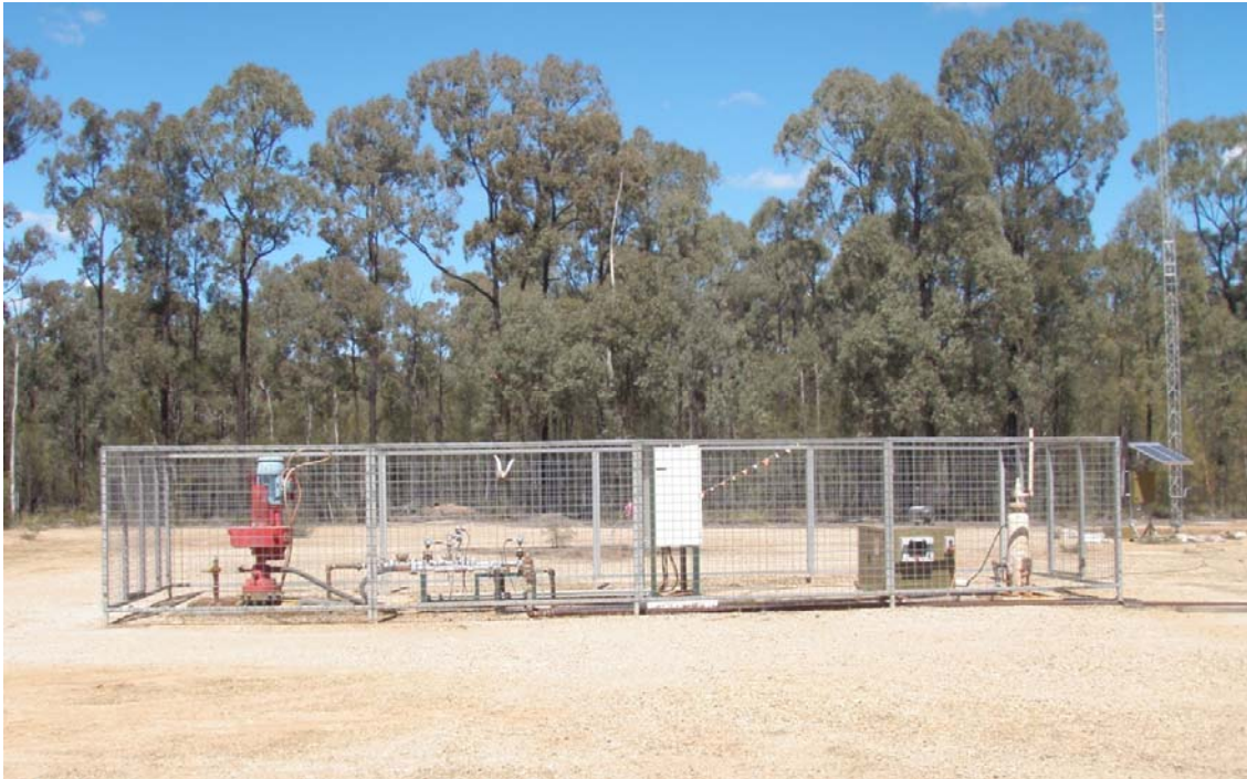
Figure 4.2: Typical surface installation required to operate a CSG well
