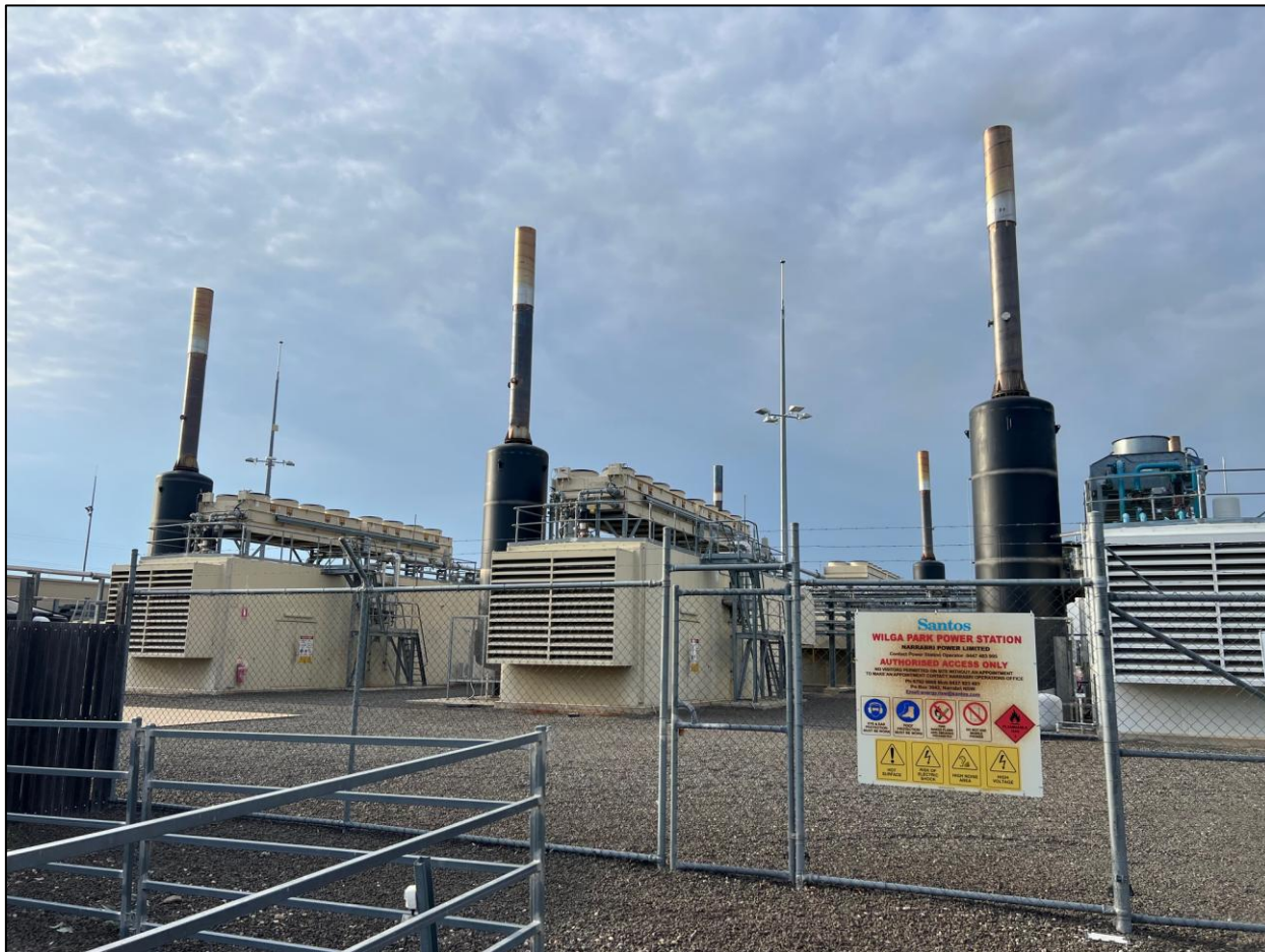
Figure 1: 3MW Generator Stack Release Points
