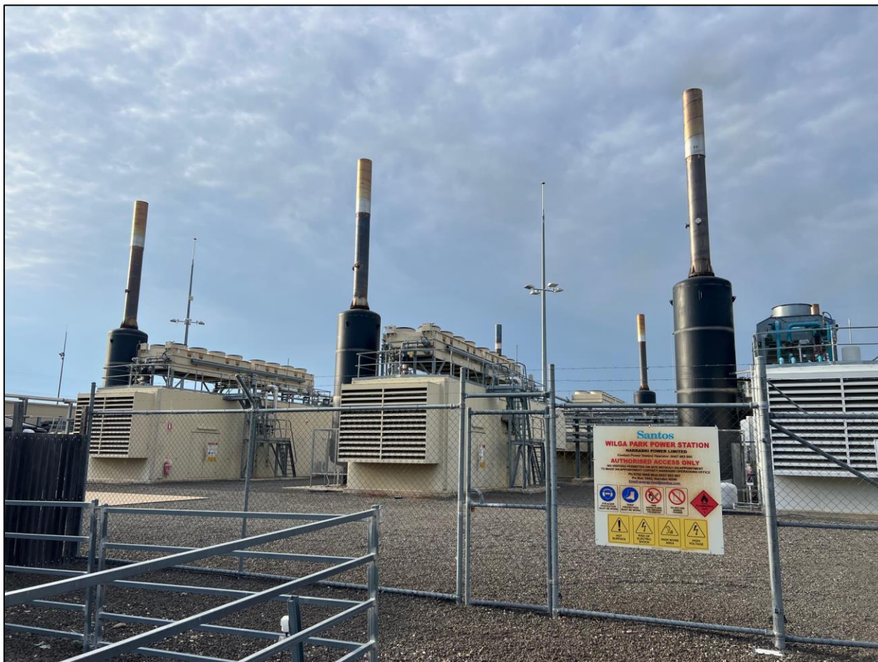
Figure 1: 3MW Generator Stack Release Points
