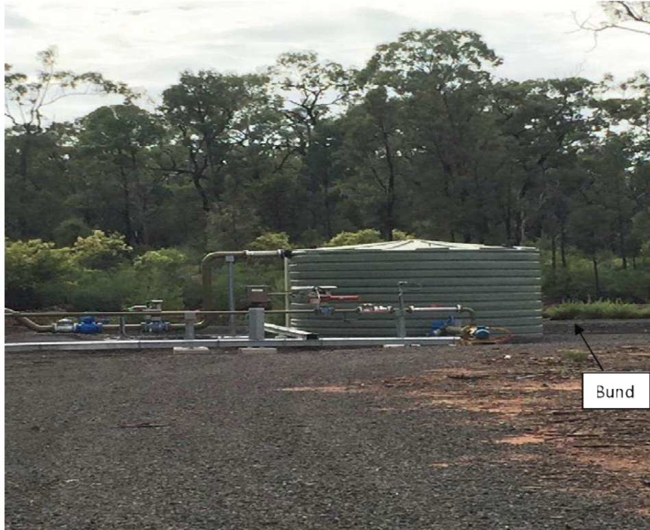
Figure 3 Dewhurst 28 – Balance tank
