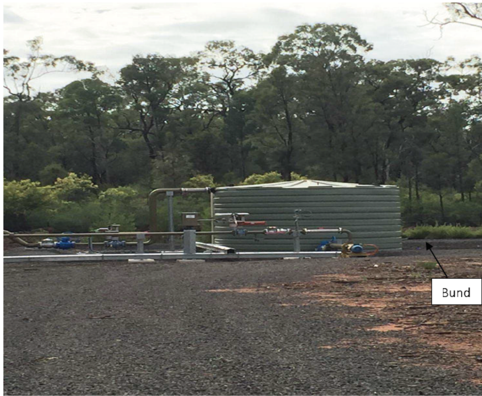
Figure 3 Dewhurst 28 – Balance tank
