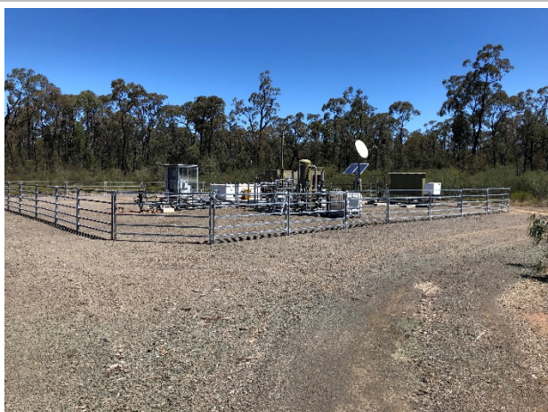
Photo 23: Dewhurst 29 – Well head and facilities
