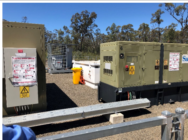
Photo 24: Dewhurst 29 – Gas and diesel generators (left/right respectively). 6,000 L diesel storage (white tank) with spill kit adjacent (yellow 240 L wheelie bin)
