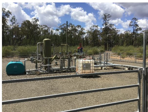
Photo 16: Dewhurst 26 – well head and facilities
