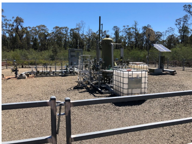
Photo 17: Dewhurst 27 – well head and facilities
