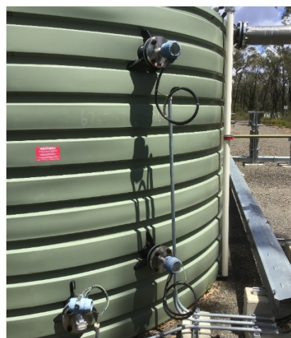
Photo 22: Dewhurst 28 – Produced water balance tank, level sensors.
