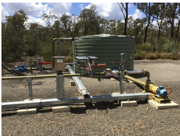
Photo 21: Dewhurst 28 – 22,000 L produced water balance tank
