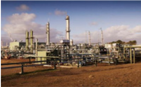
Iona gas plant, VIC
