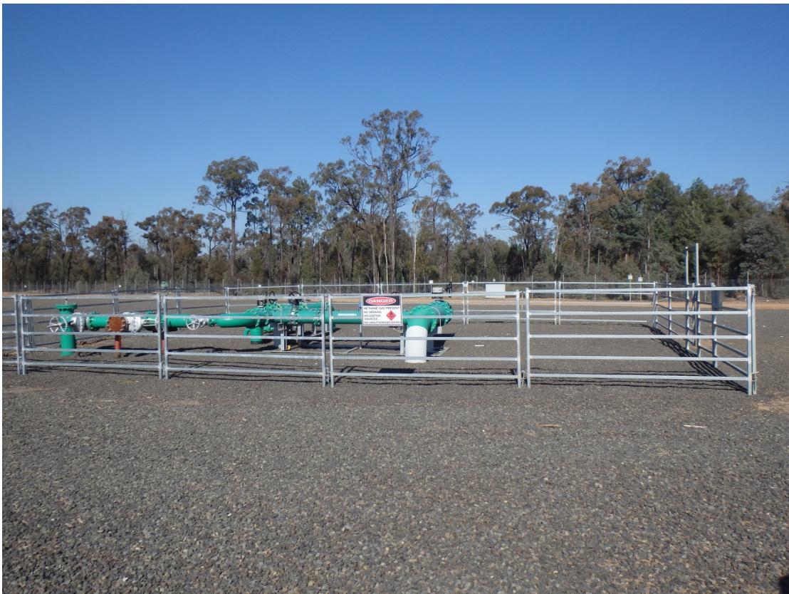
Plate 2 – Bibblewindi inlet manifold and associated pipework
