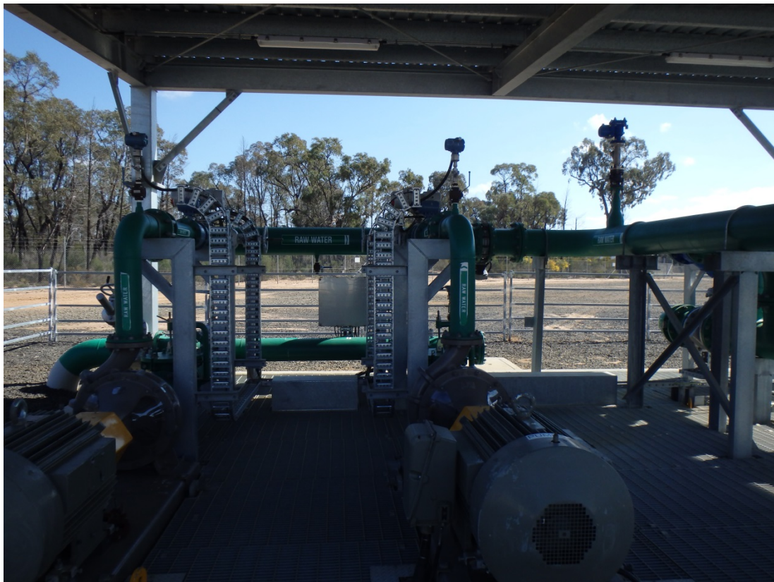
Plate 3 – Biblewindi outlet manifold, associated pumps, pipework and metering equipment
