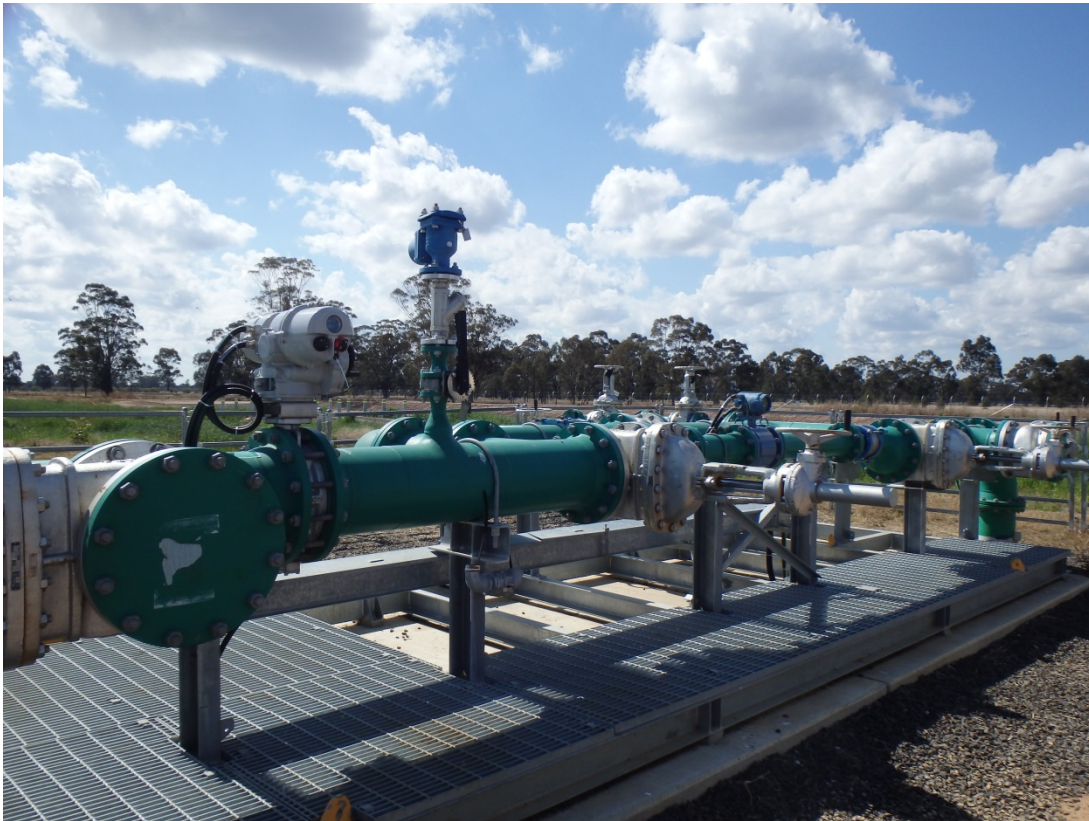
Plate 9 – Leewood inlet manifold and associated pumps and metering equipment
