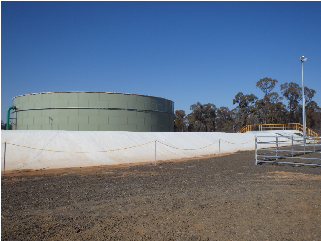
Plate 1 – 5ML tank at the Bibblewindi Facilities Area
