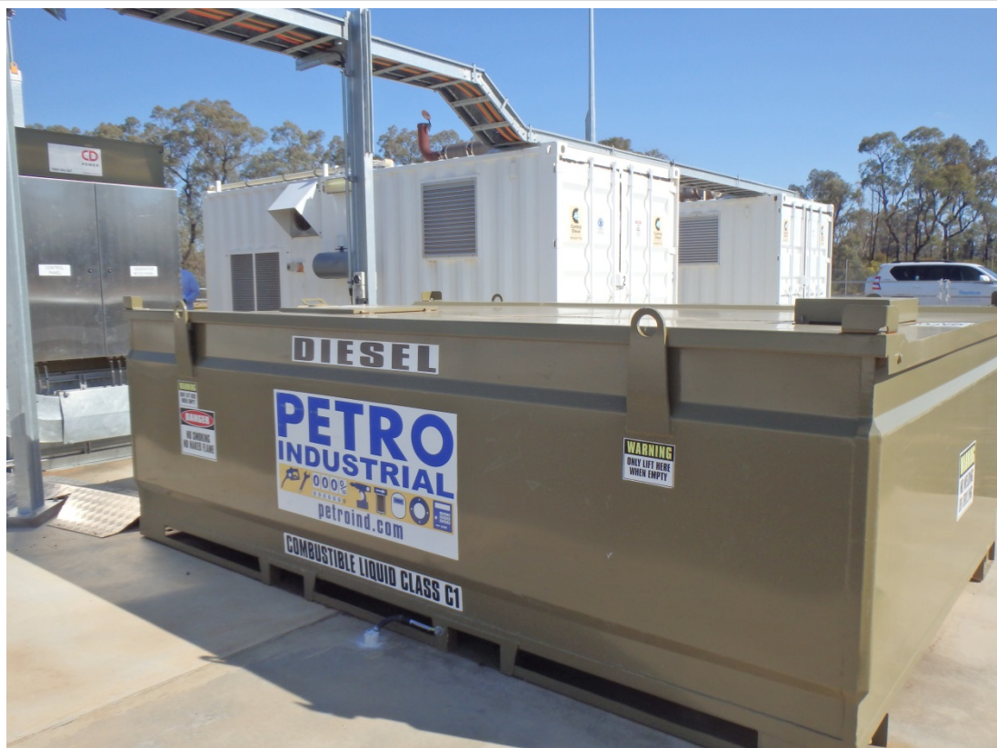
Plate 4 – Biblewindi gas fired engines and backup diesel generator
