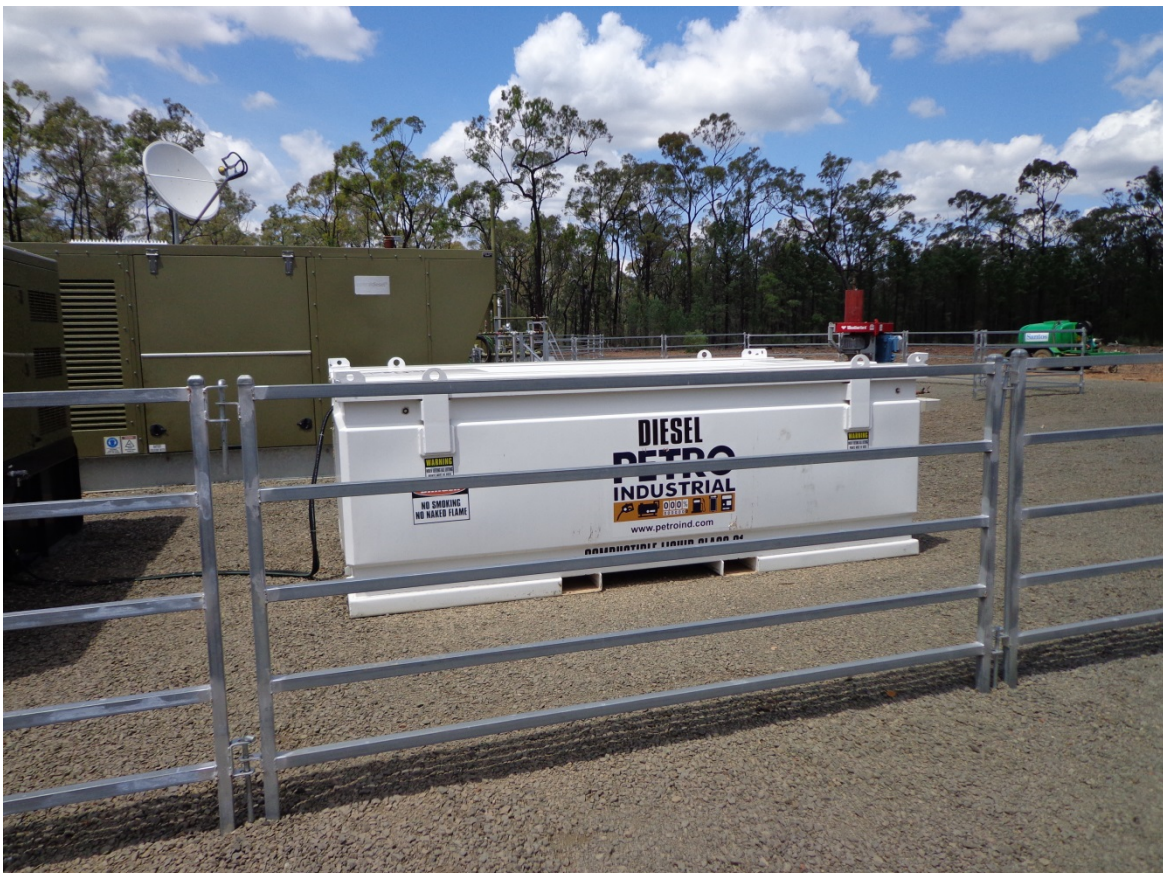
Diesel storage container at Dewhurst 28
