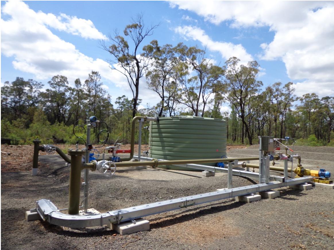
Dewhurst 28 produced water collection and transfer tank
