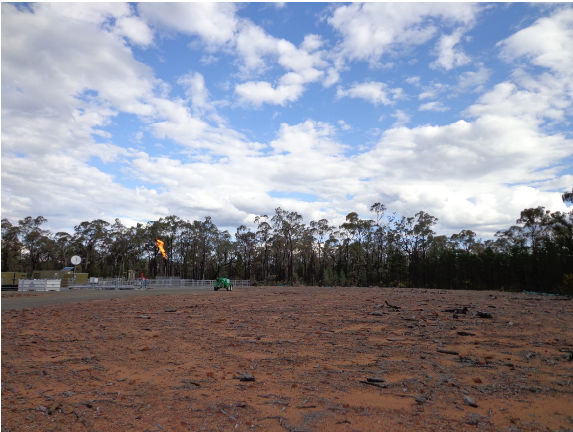
Dewhurst 28 flare and well head
