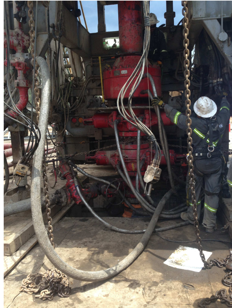
Well head infrastructure during drilling, Santos Narrabri
