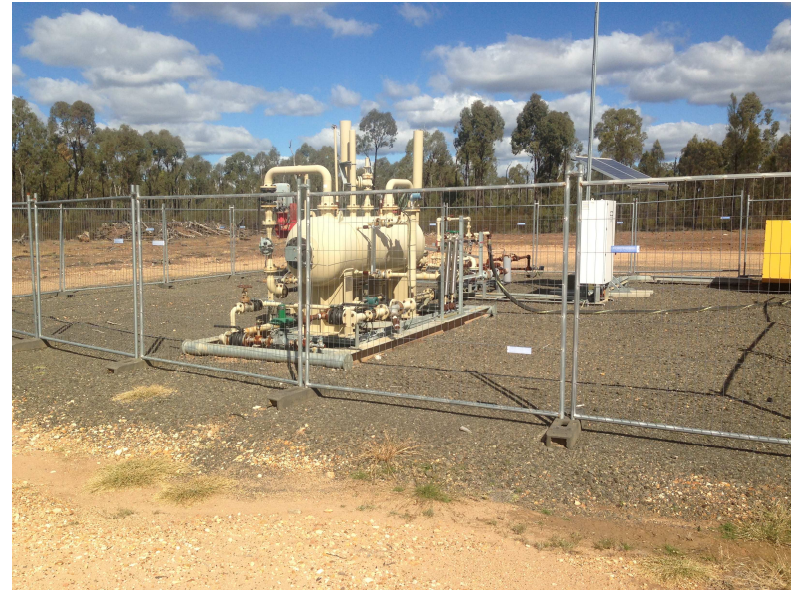
Well head infrastructure following drilling prior to partial rehabilitation, Santos Narrabri
