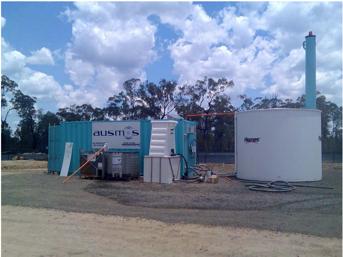
Figure 4 Reverse Osmosis pilot located at Bibblewindi-1
