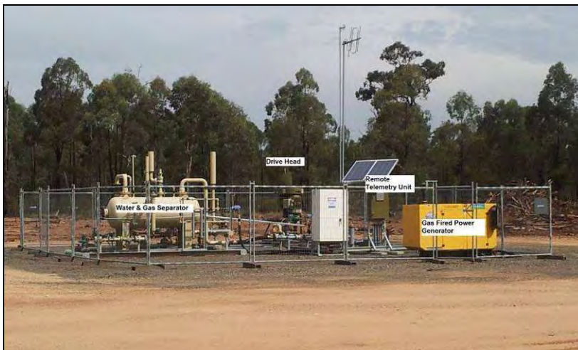
Figure 1.2.3.1 - Typical wellhead for extraction of gas and CSG water from coal seams
