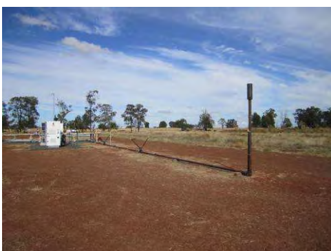
Figure 1.2.3.2: Typical flare assembly
