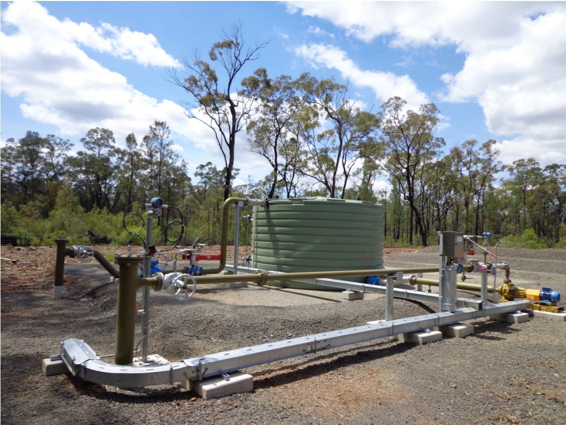
Dewhurst 28 produced water collection and transfer tank
