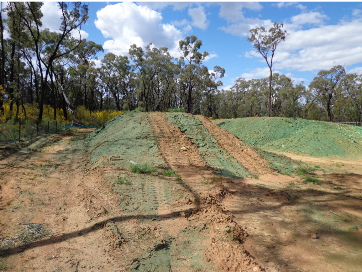
Dewhurst 31 topsoil stockpile showing disturbed polymer seal
