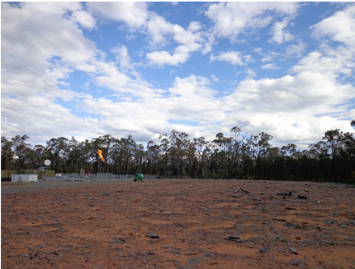
Dewhurst 28 flare and well head
