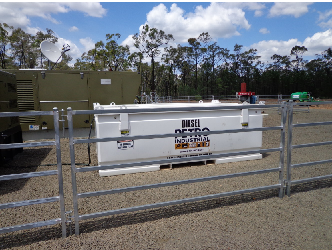
Diesel storage container at Dewhurst 28
